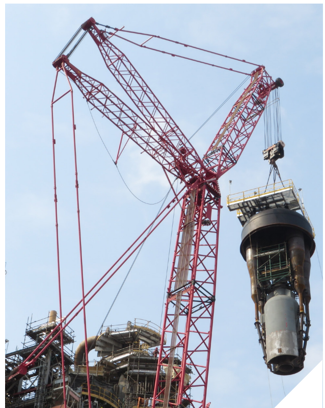
Installation of this riser termination device in the reactor reduced coke and dry gas and improved product yield selectivity.
